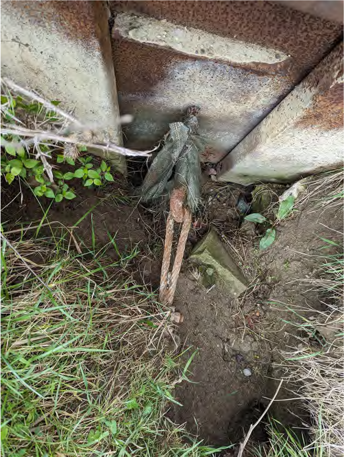
PHOTO NO. 3: Harbor Island Center tie exposed.
