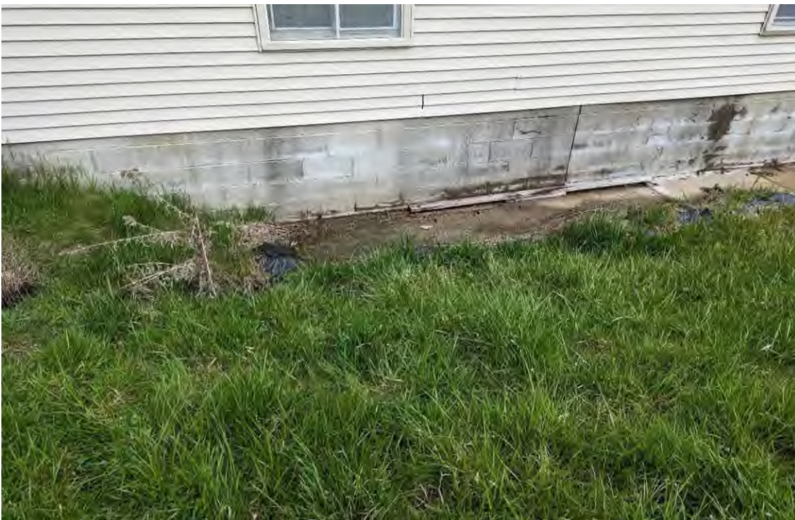
PHOTO NO. 6: Harbor Island Center north covered dock with indication of settlement.
