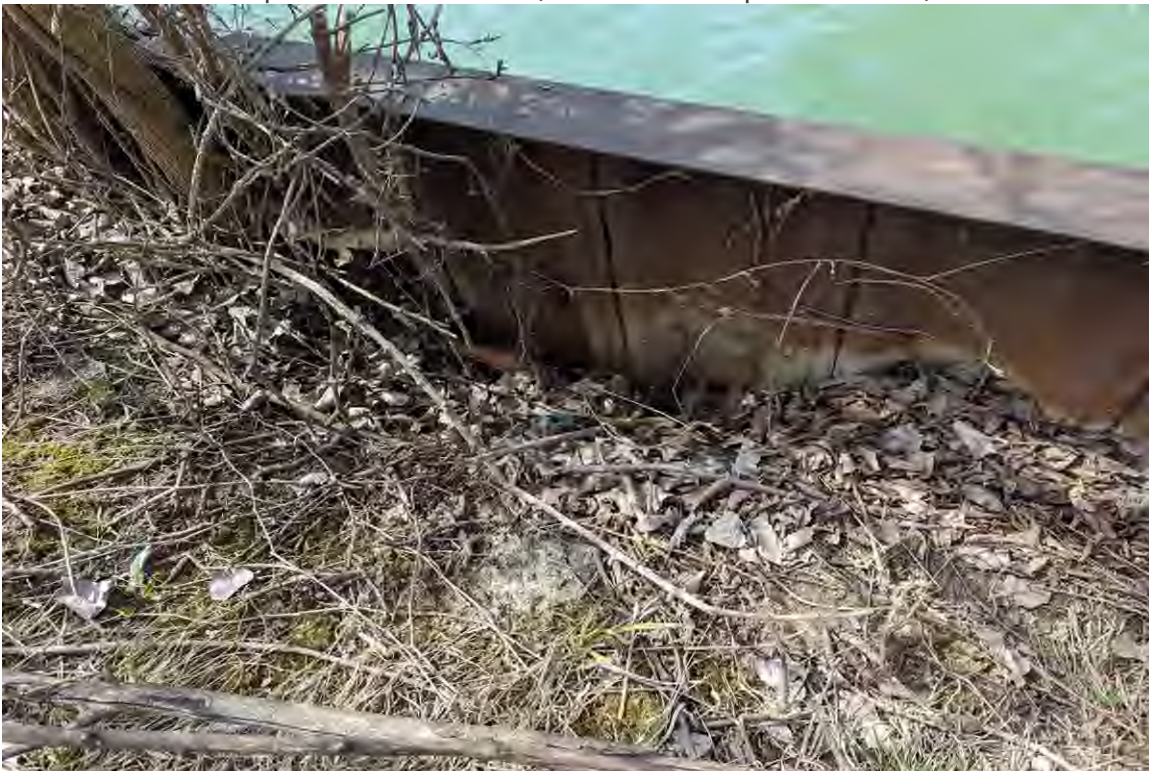
PHOTO NO. 12: Exposed Anchor Rod and Soil Settlement
