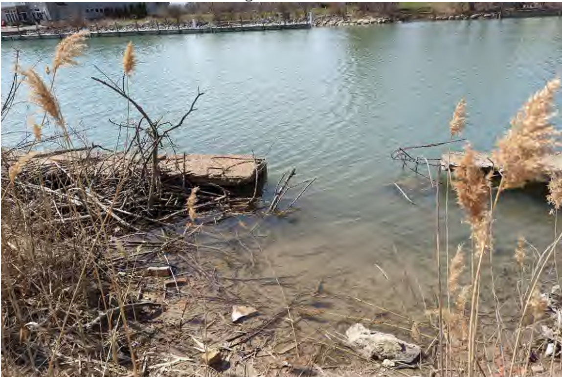
PHOTO NO. 4: Eroded Concrete Seawall
