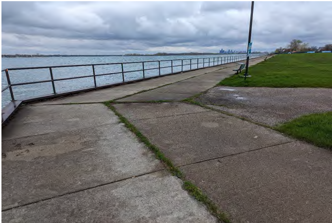
PHOTO NO. 2: Sidewalk at upriver corner.
