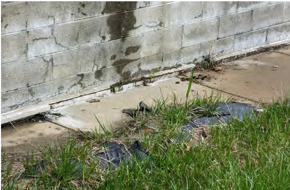
PHOTO NO. 7: Cracked masonry block of north covered dock.
