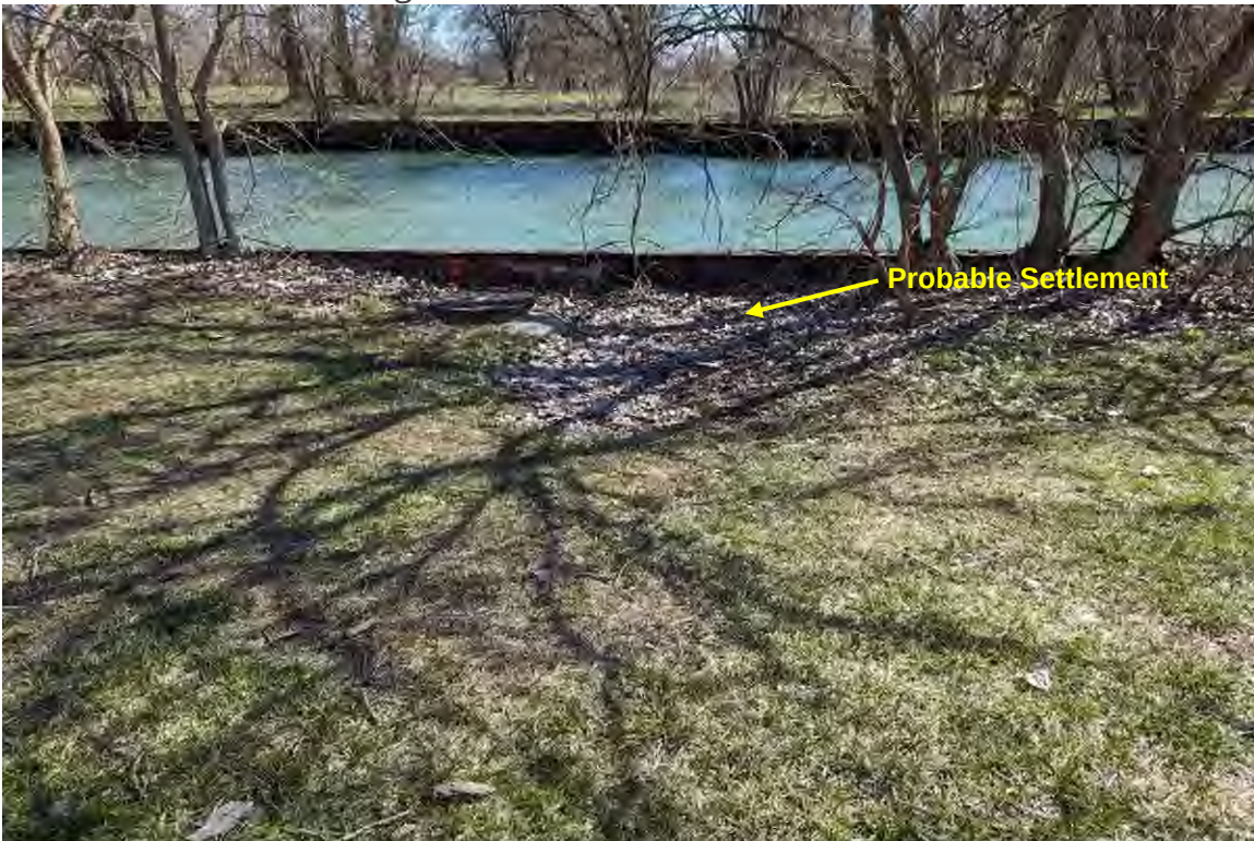
PHOTO NO. 4: Possible soil migration into manhole or into channel
