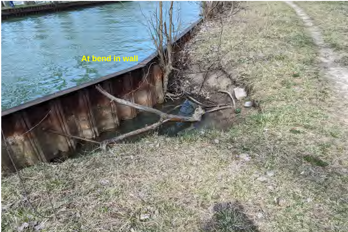
PHOTO NO. 13: Exposed Anchor Rod and Erosion behind wall.
