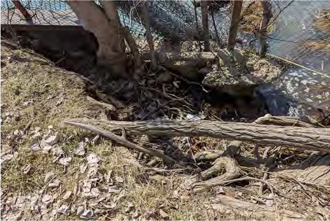
PHOTO NO. 1: Erosion due to failed concrete seawall on adjacent property.
