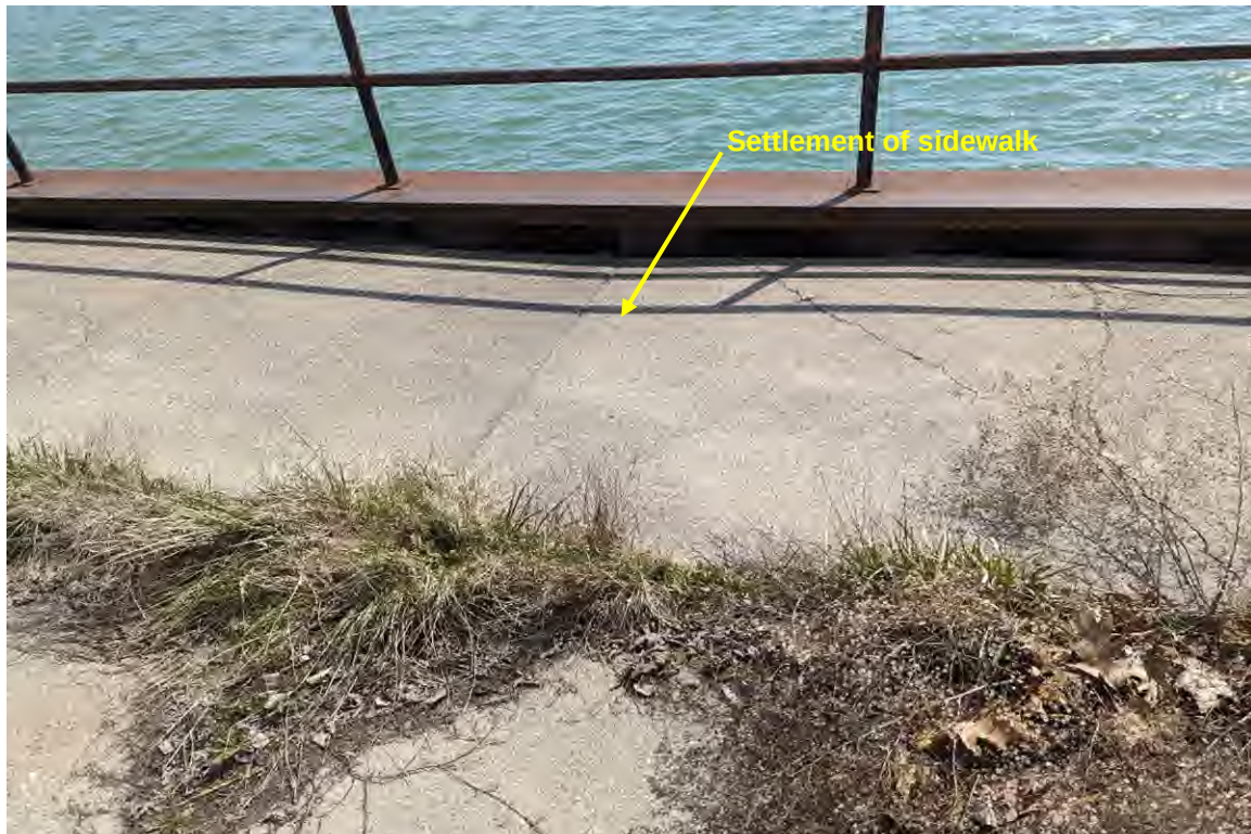
PHOTO NO. 5: Sidewalk settlement
