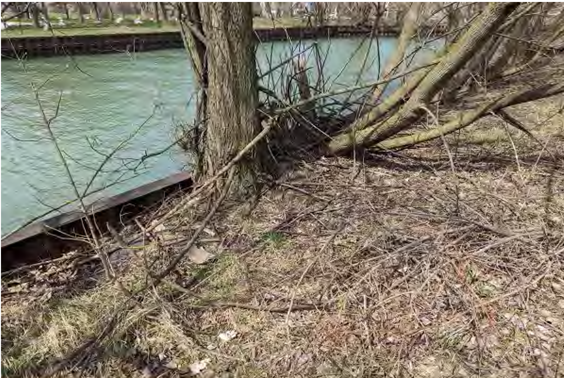
PHOTO NO. 10: Trees adding stress to seawall (along entire channel)
