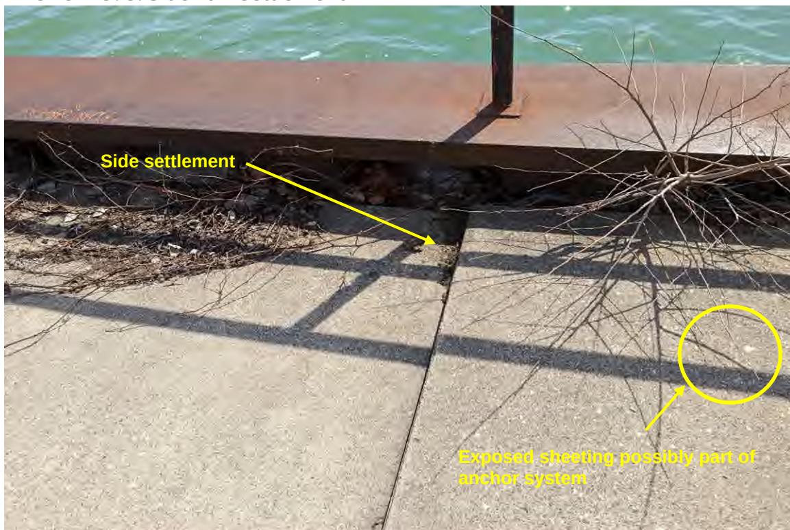
PHOTO NO. 6: Sidewalk settlement
