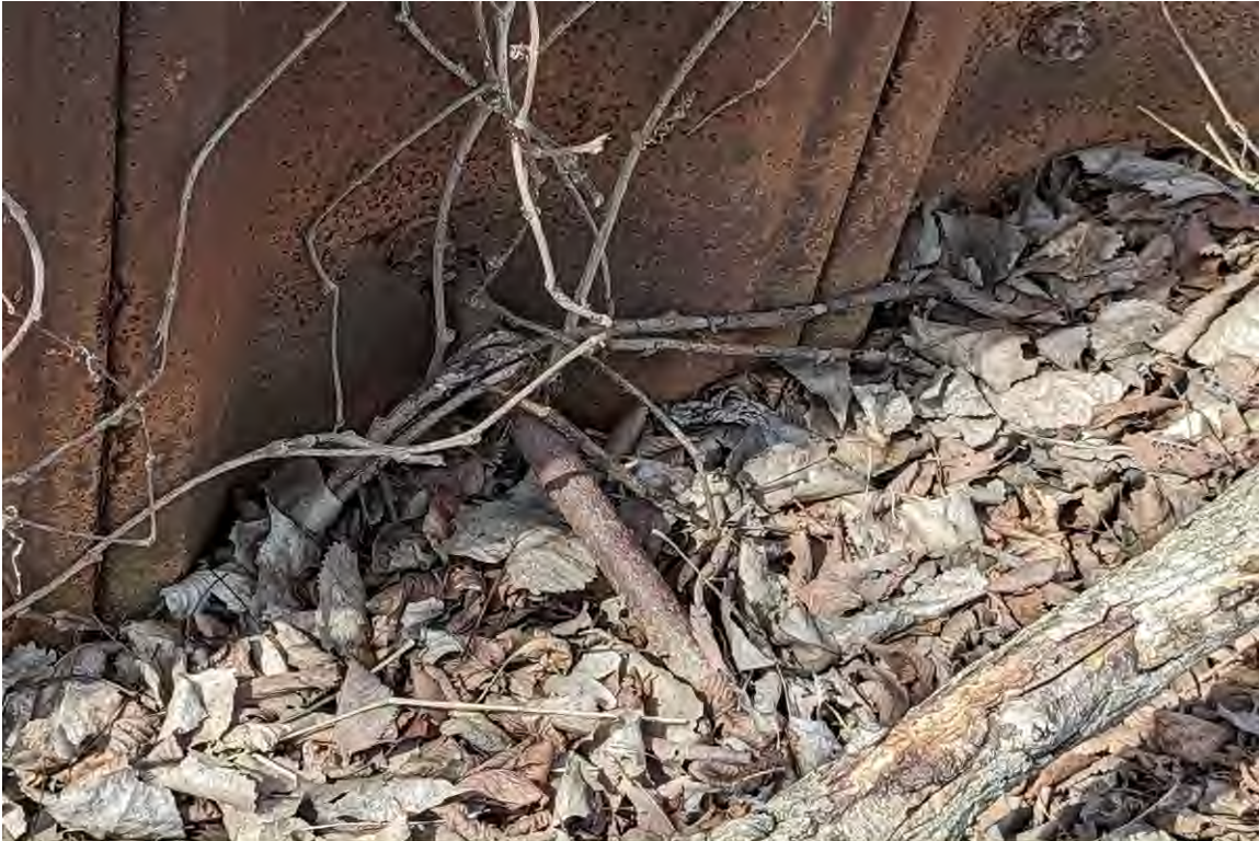
PHOTO NO. 11: Exposed Anchor Rod (noted in multiple locations)
