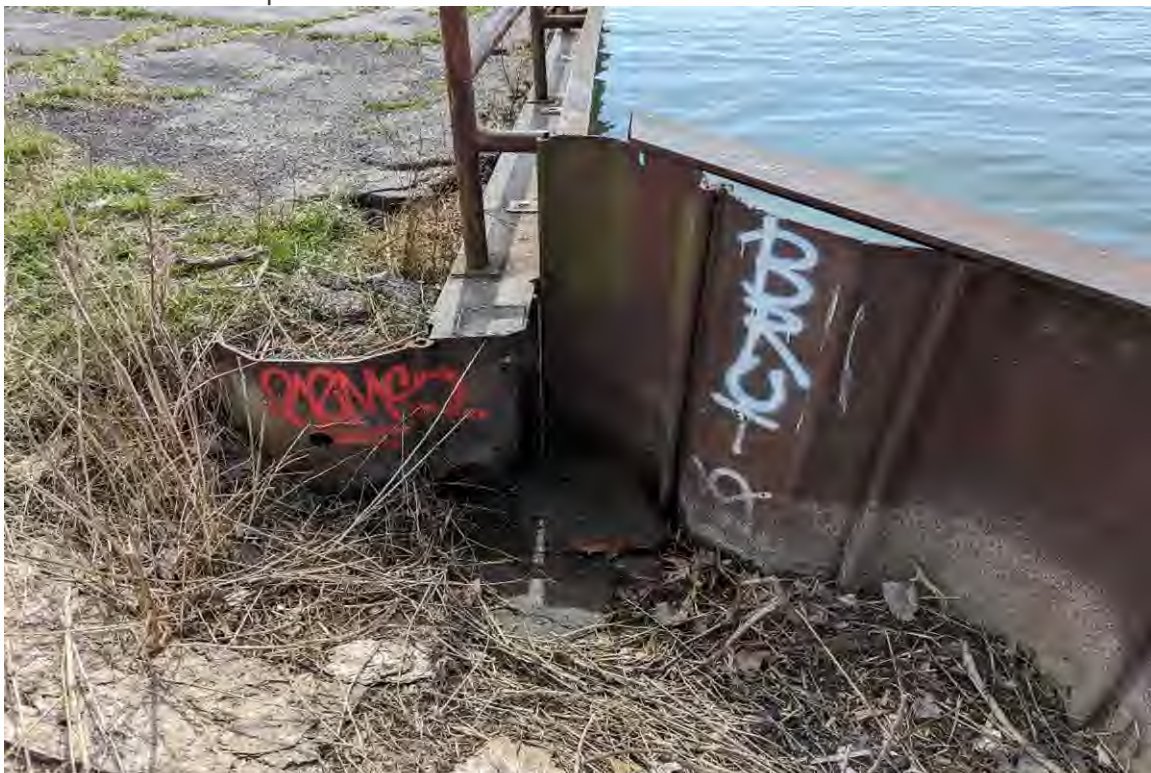
PHOTO NO. 14: Erosion behind sheeting at interface
