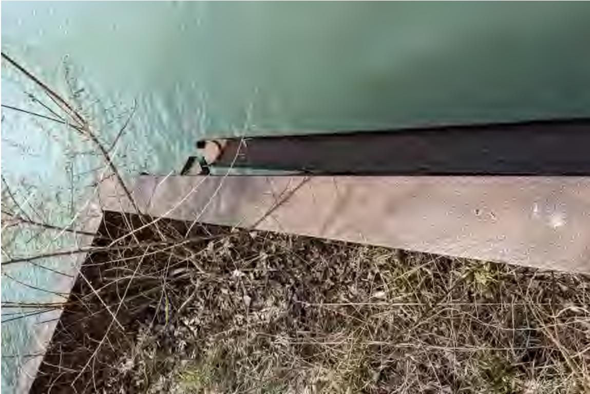
PHOTO NO. 9: Broken Whaler Connection
