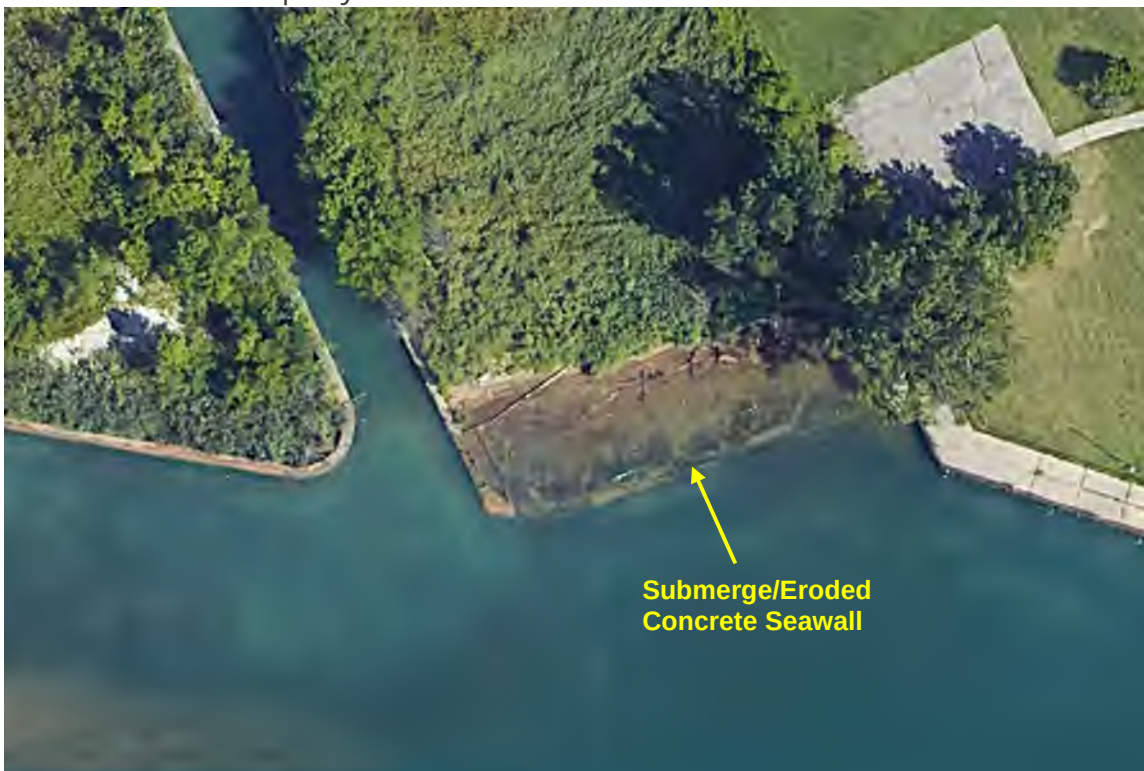
PHOTO NO. 24: Eroded Seawall
