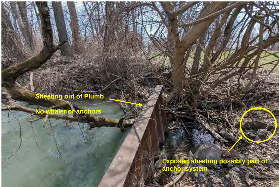
PHOTO NO. 6: Erosion behind sheeting
