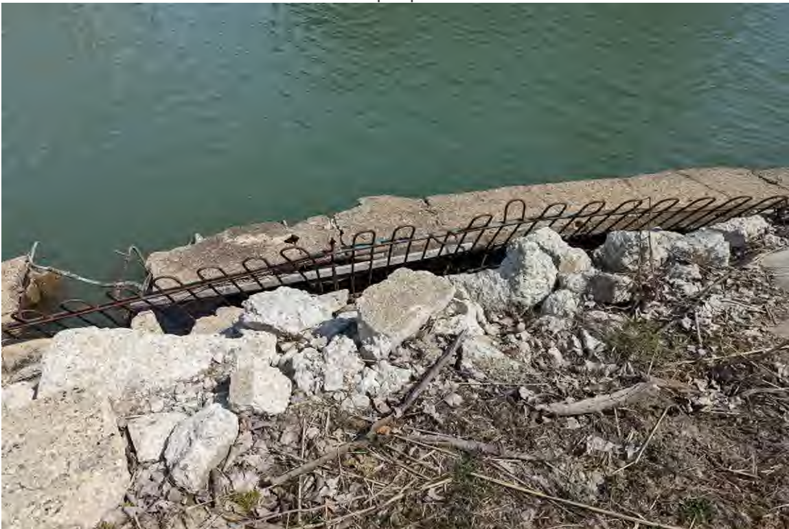
PHOTO NO. 2: Failed original concrete seawall
