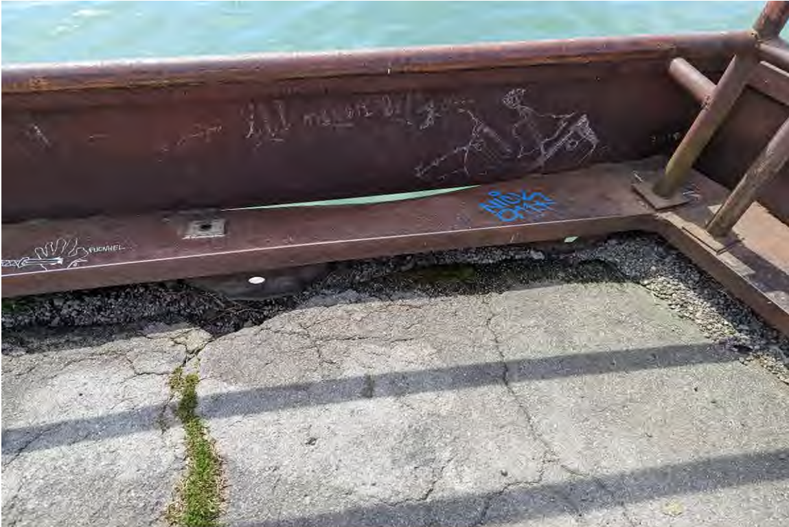
PHOTO NO. 15: Bent metal ledge and settlement of pavement.
