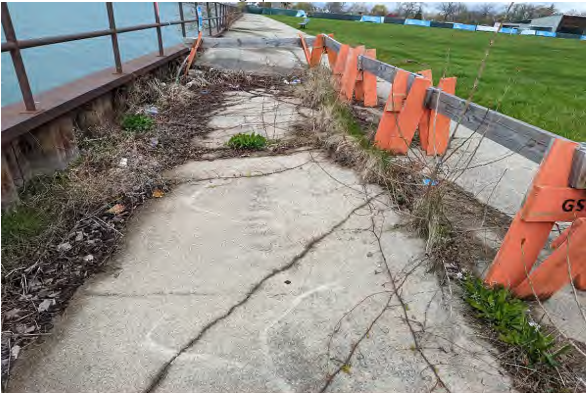
PHOTO NO. 6: Wall failure looking down river.
