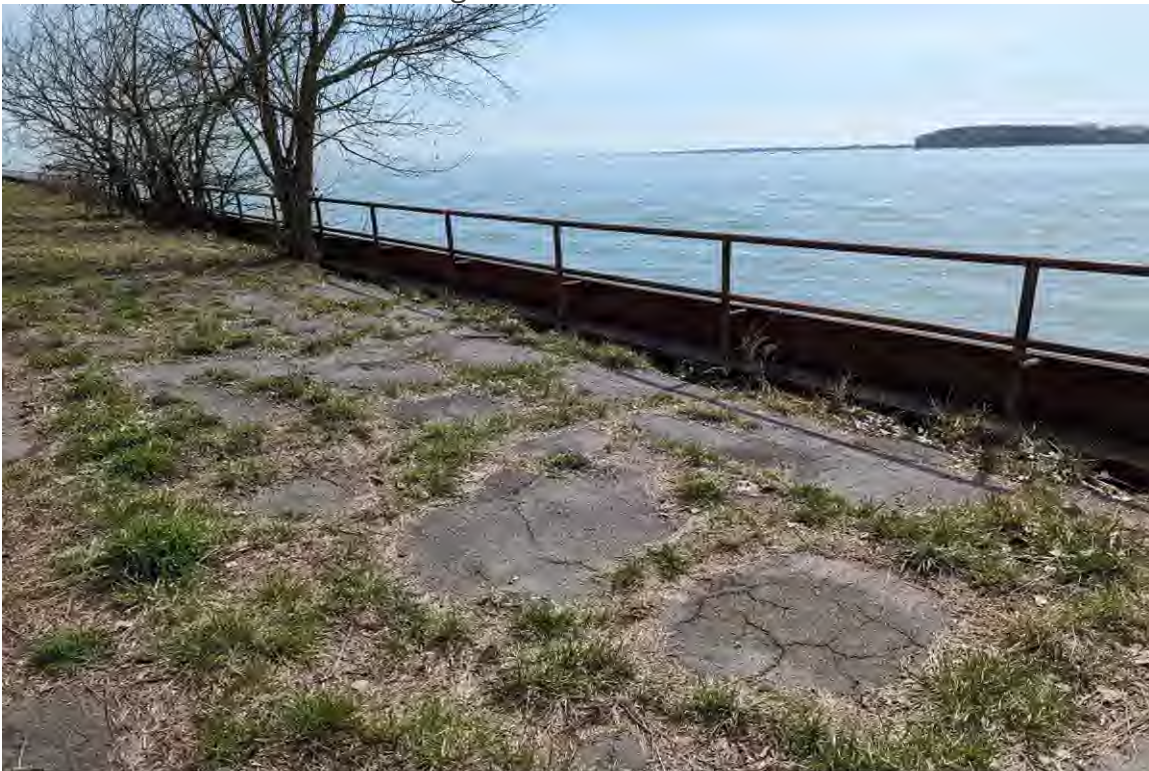
PHOTO NO. 18: Pavement failure and being overgrown.
