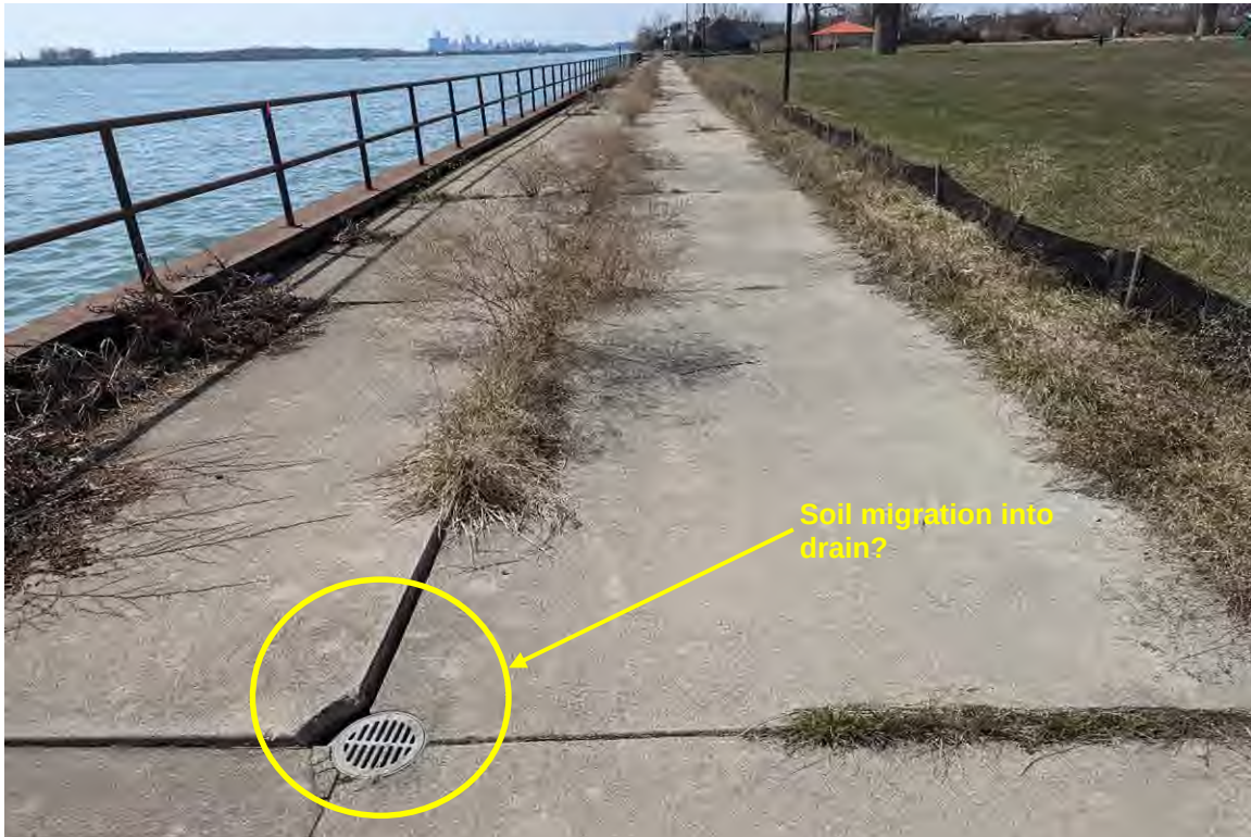
PHOTO NO. 7: Soil migration into drain
