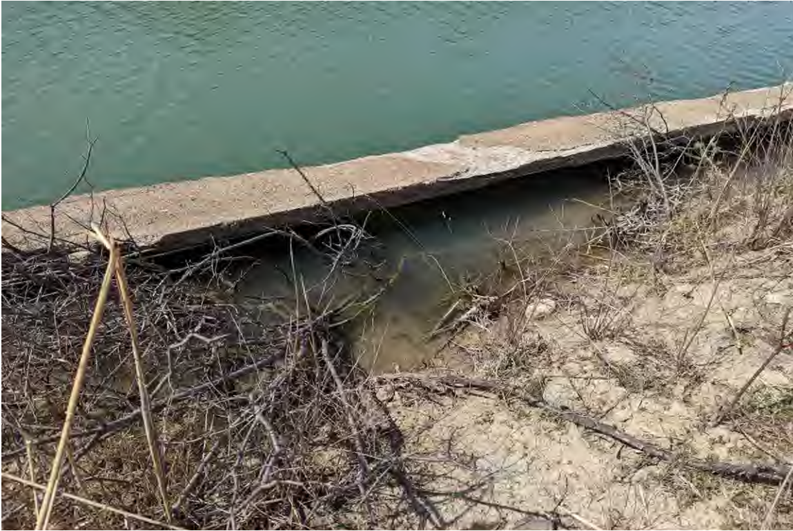
PHOTO NO. 1: Eroded and undermined seawall along channel
