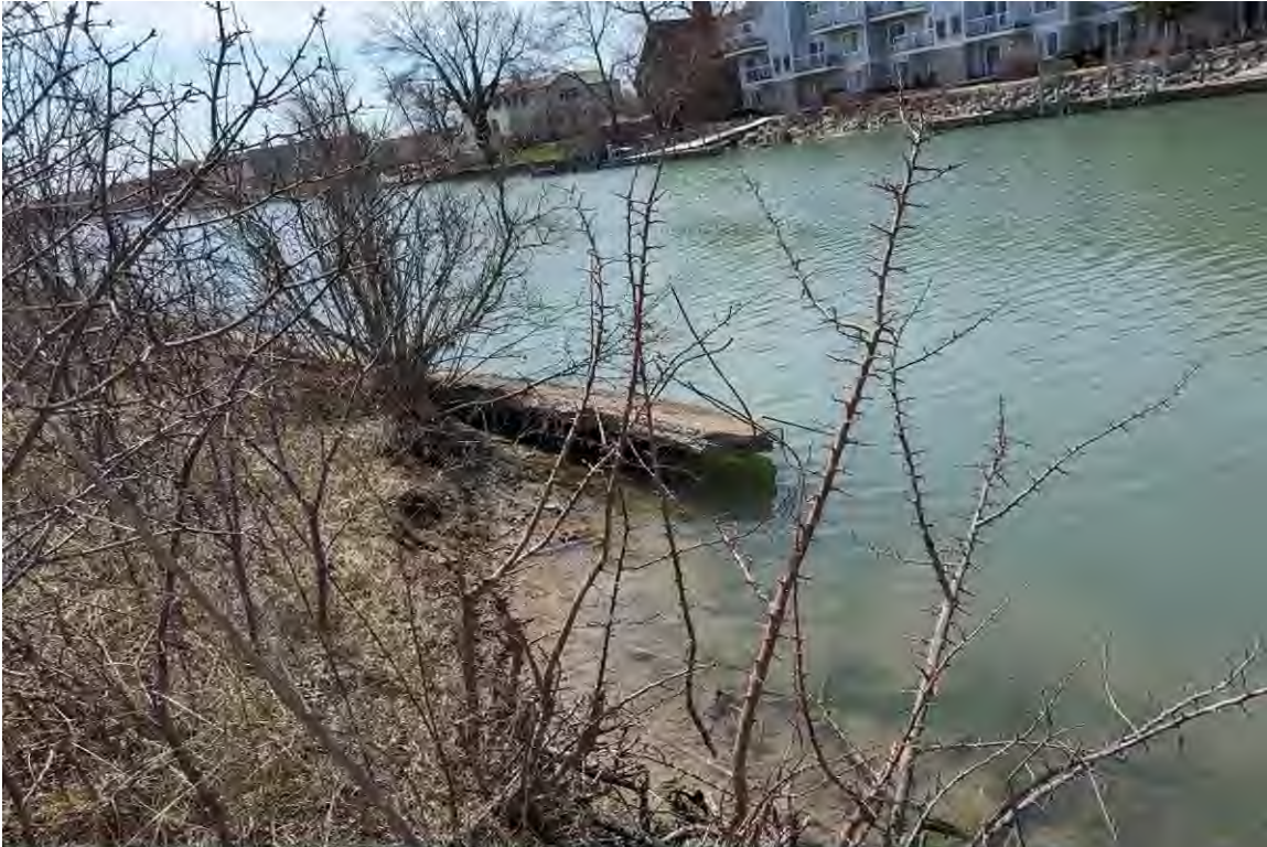
PHOTO NO. 3: Eroded Seawall along Channel
