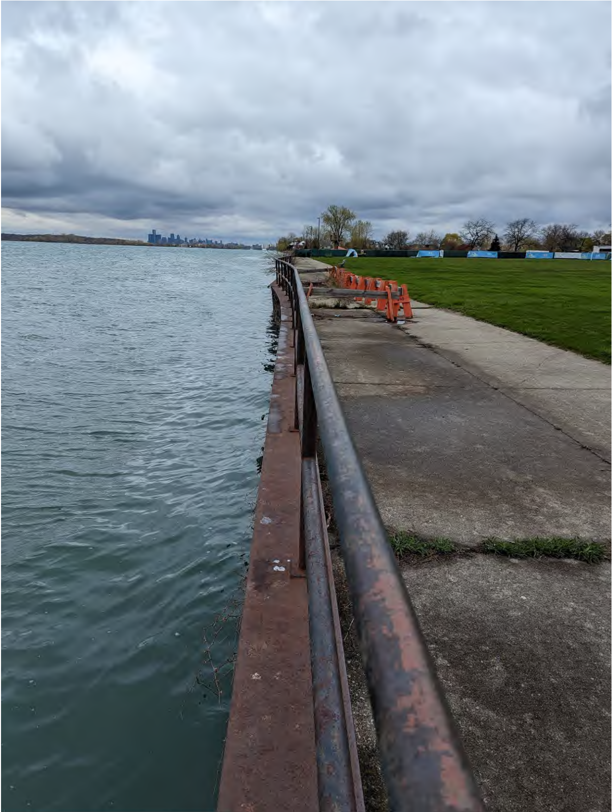
PHOTO NO. 8: Wall failure looking down river.
