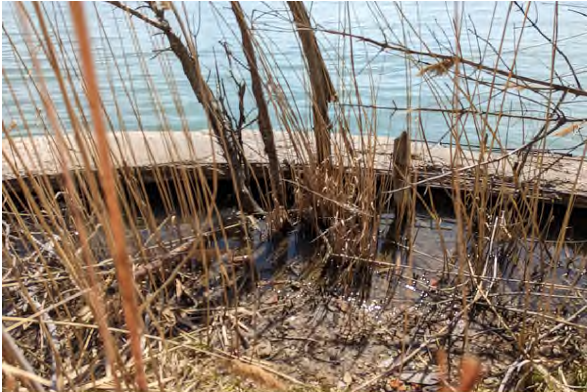
PHOTO NO. 21: Eroded Concrete Seawall
