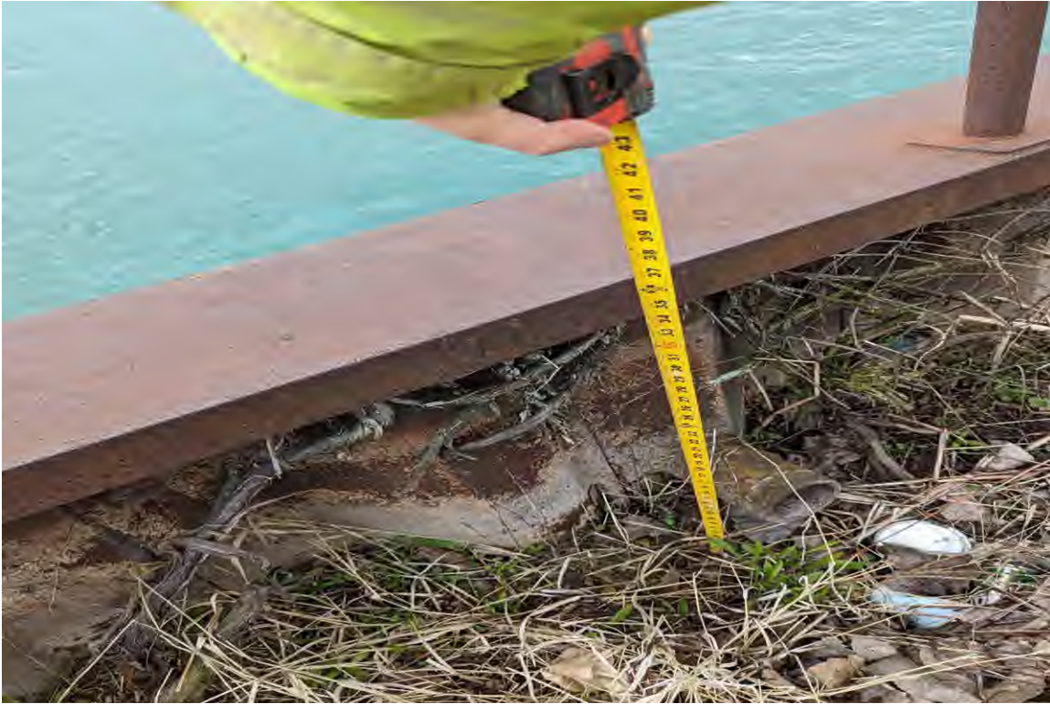
PHOTO NO. 7: Settlement behind wall failure.
