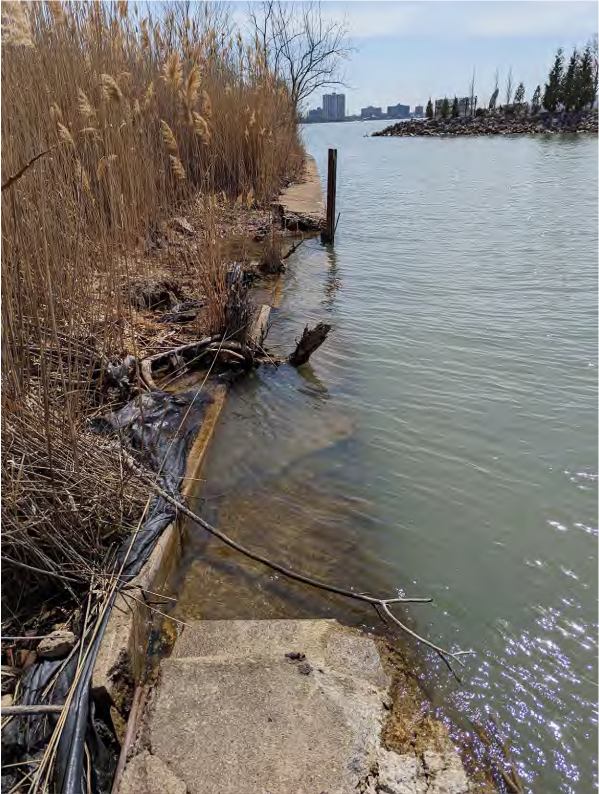
PHOTO NO. 16: Eroded Concrete Seawall
