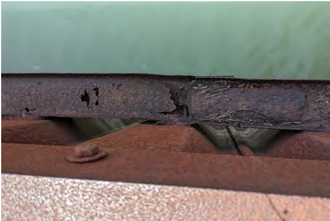
PHOTO NO. 8: Whaler completely rusted through. (Noted in multiple locations)
