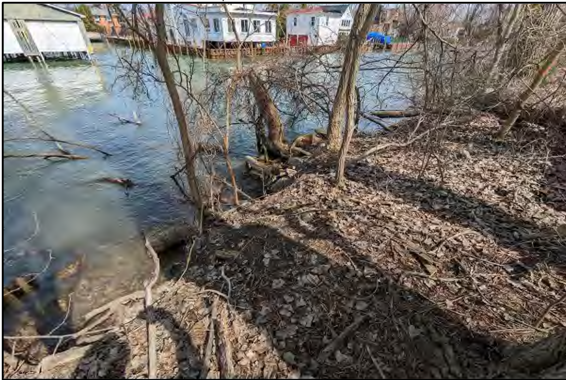
PHOTO NO. 2: Erosion of channel bank with no rip-rap present
