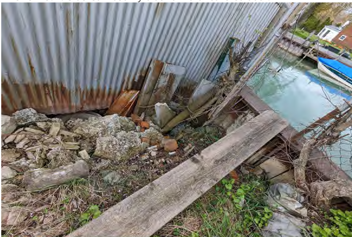
PHOTO NO. 8: Concrete and steel debris at interface between seawall and south dock.
