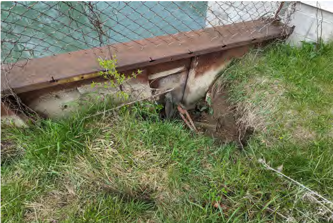
PHOTO NO. 2: Harbor Island Center exposed tie.
