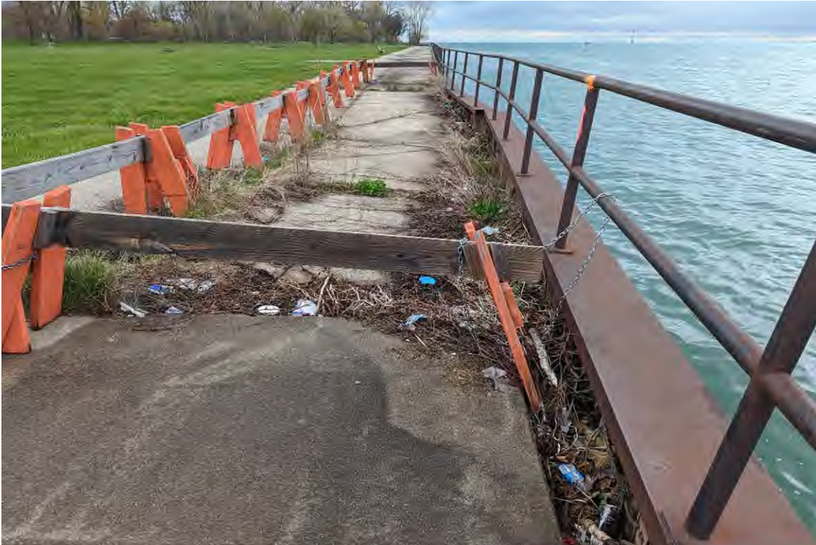
PHOTO NO. 5: Wall failure looking upriver.
