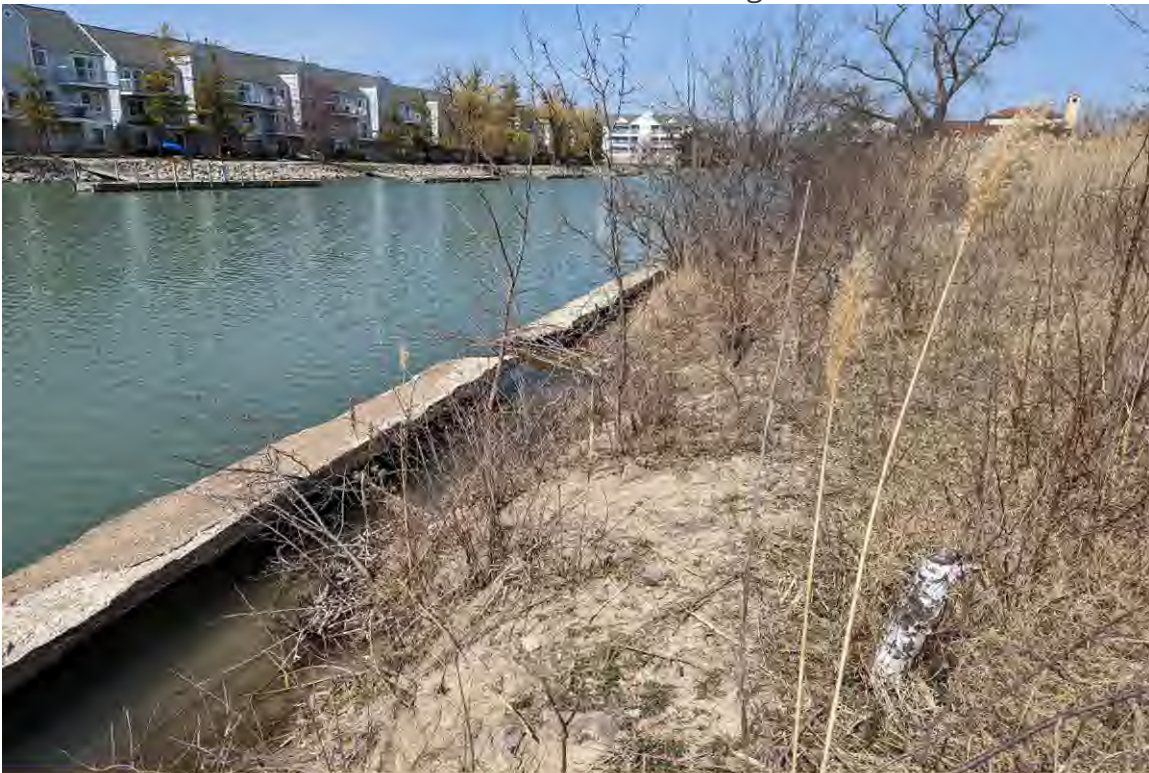
PHOTO NO. 2: Eroded and undermined seawall along channel
