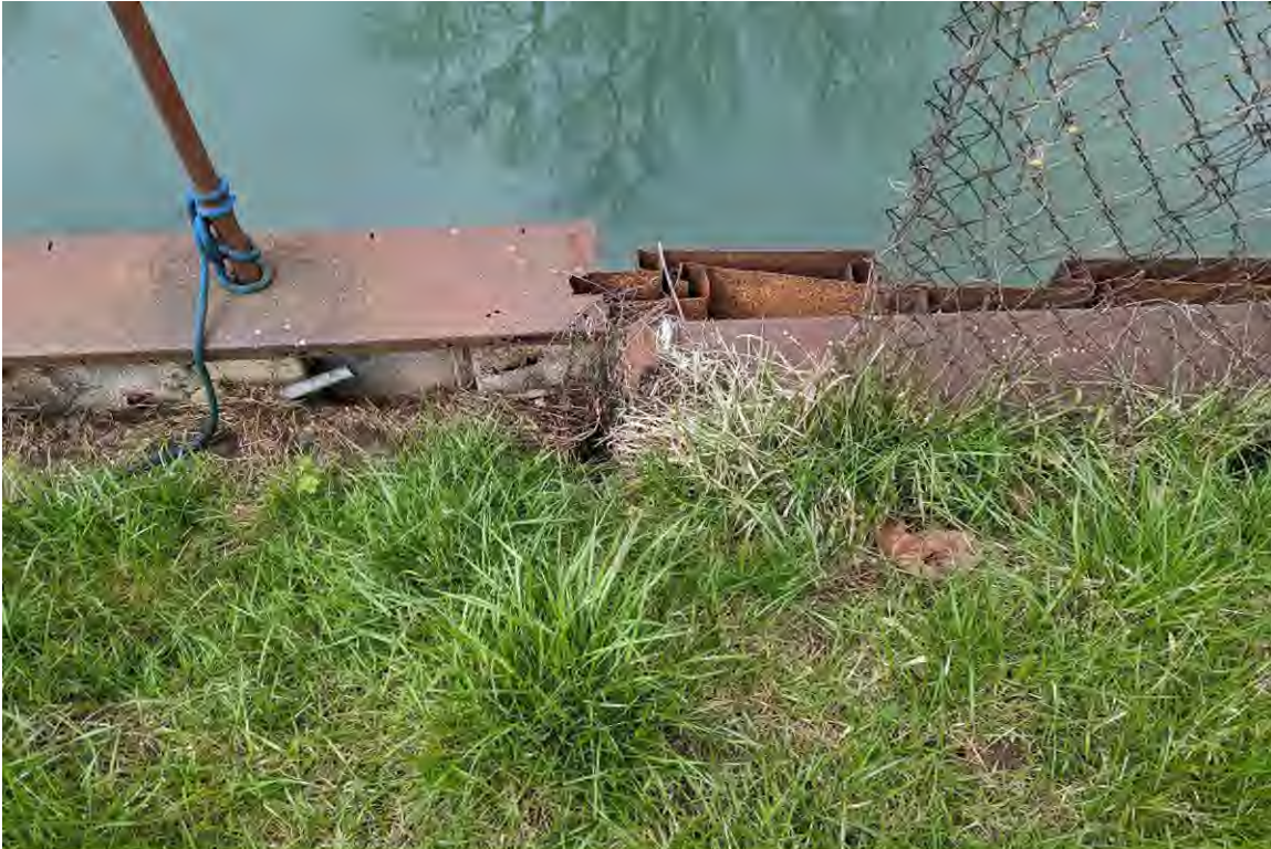
PHOTO NO. 1: Harbor Island Center seawall failure from above.
