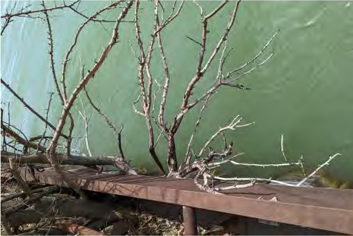
PHOTO NO. 19: Tree growing through Sheeting
