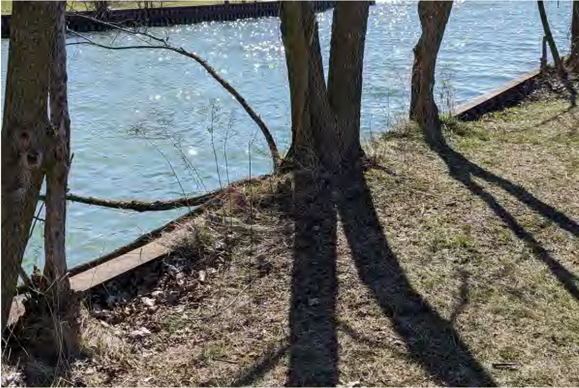
PHOTO NO. 5: Overgrown trees causes increased stress on wall and anchors.
