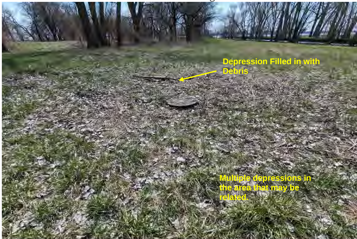
PHOTO NO. 4: Possible soil migration into manhole
