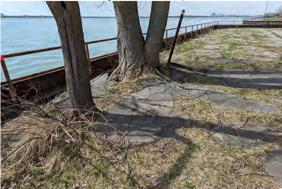
PHOTO NO. 16: Tree Disturbing Pavement and Possibly Sheeting
