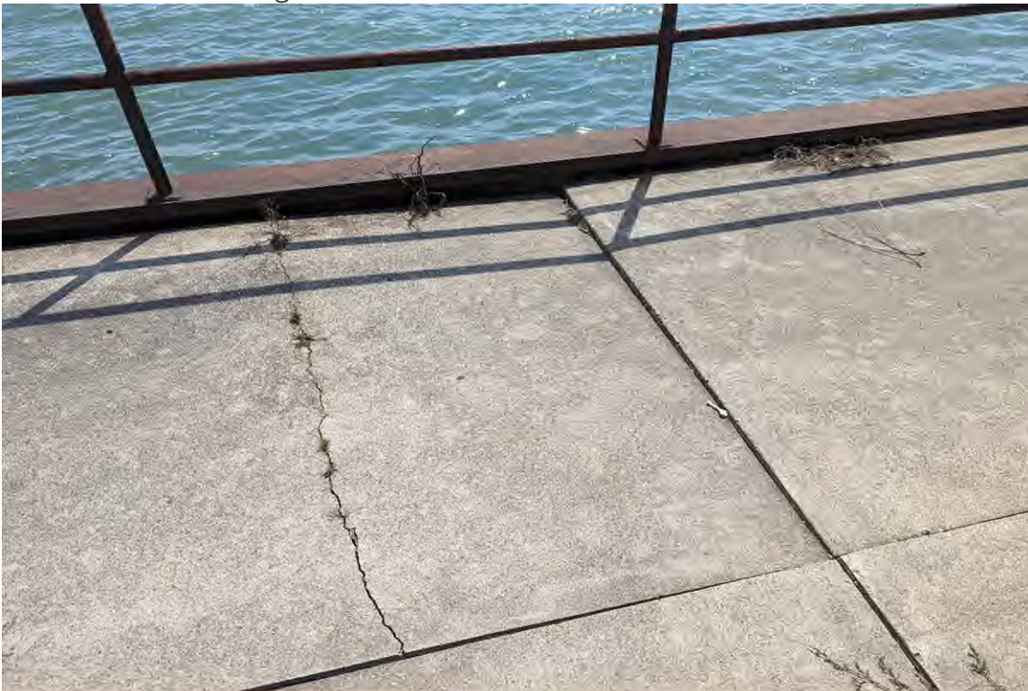
PHOTO NO. 8: Sidewalk settlement
