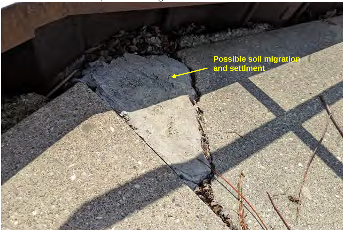
PHOTO NO. 4: Possible soil migration into river.
